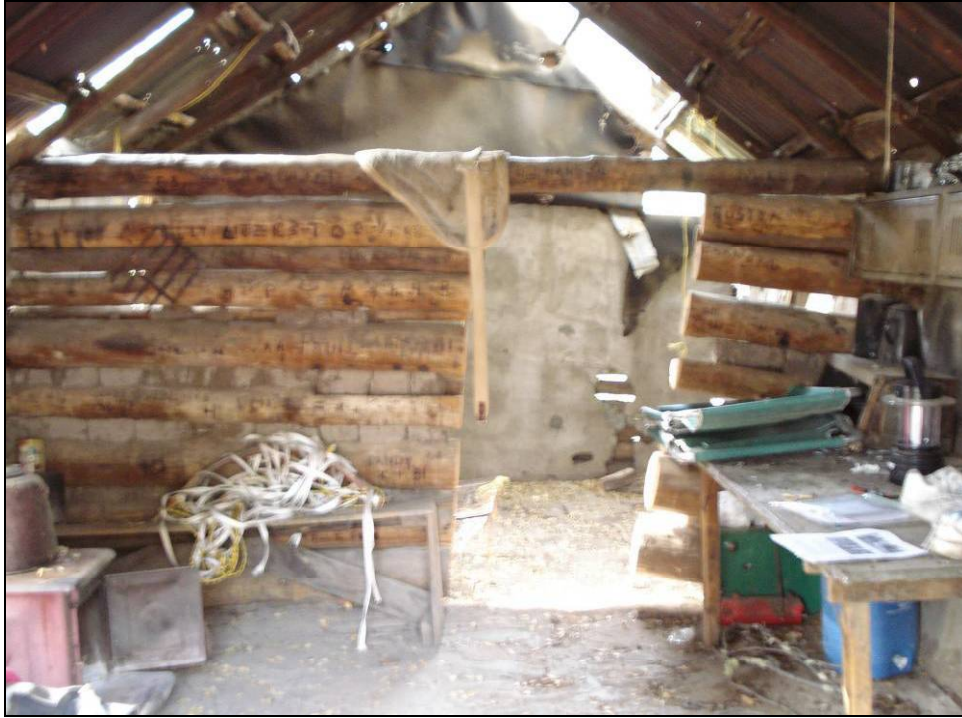
Photograph B-7. Overview of the interior showing the doorway cut in the structural wall between the pens and the movement of the logs on the west (right), looking south. Photograph date: 6 May 2009.
