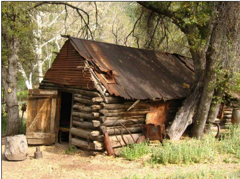
Photograph B-6. Exterior view of the west wall of the Tony Ranch cabin, which is partially supported by a tree. View looking southeast. Photograph date: 6 May 2009.
